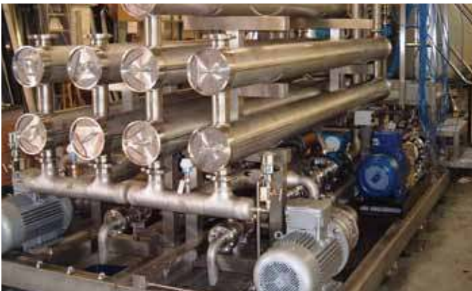
Pumping for waste stream reduction and salt solution concentration at a pharmaceutical chemical plant
